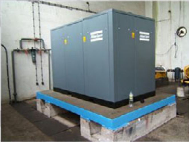
Name: Atlas - Copco Type: 4352 Manufacture: Atlas - Copco Capacity 25 m3/h Compressor 4352 Work pressure 9 atm. Year of production 2003 Number of compressors: 2
